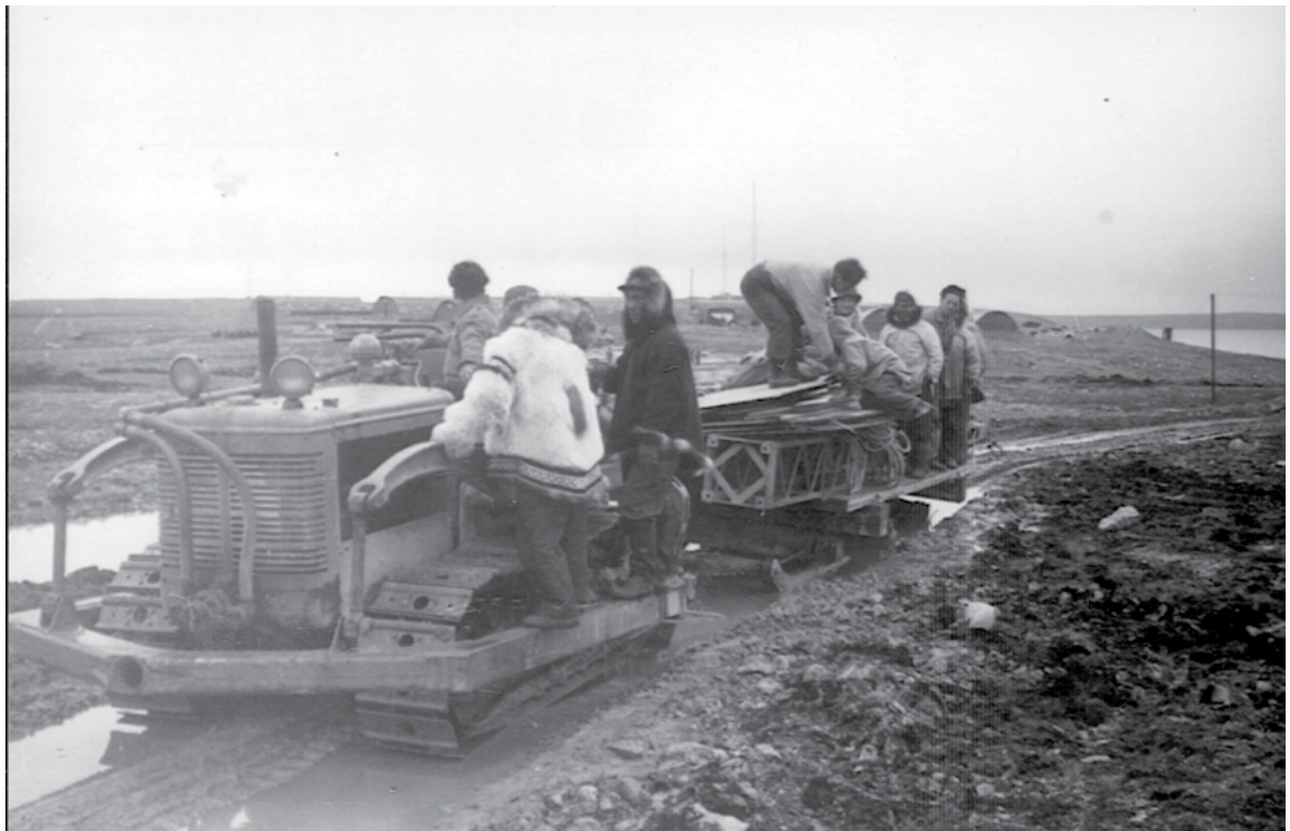
Construction of the LORAN tower in Cambridge Bay, 1947. Photographer unknown. On file at PI/KHS archives.
